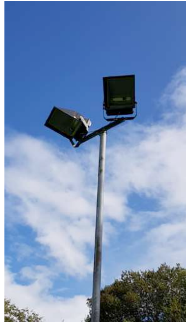
Damaged floodlights to be replaced with new energy efficient, unobtrusive flood lighting
