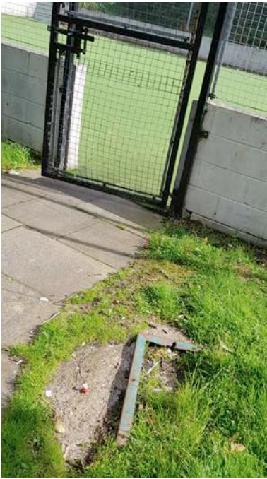
Damage to gate to be repaired and exposed metal work on ground at entry to be removed
